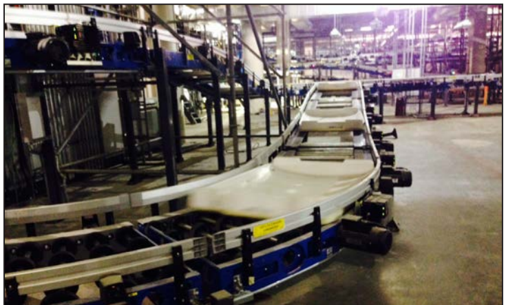
Above: Tote-Tray conveyor system
